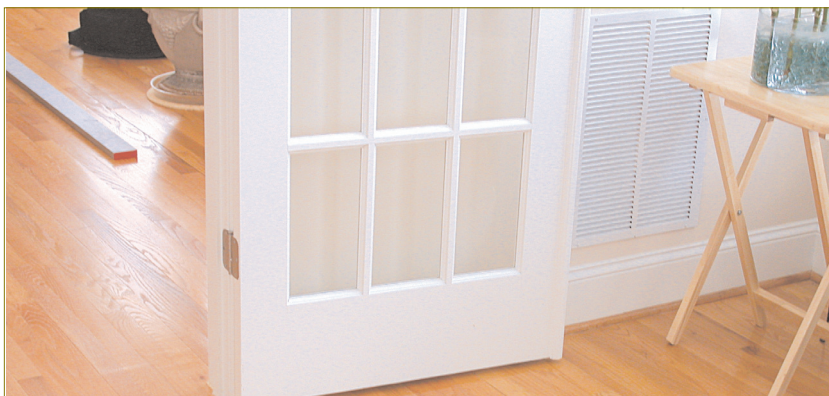
Note gap under door and near straight edge. There is a gap in both rooms along the subfloor panel edge.
